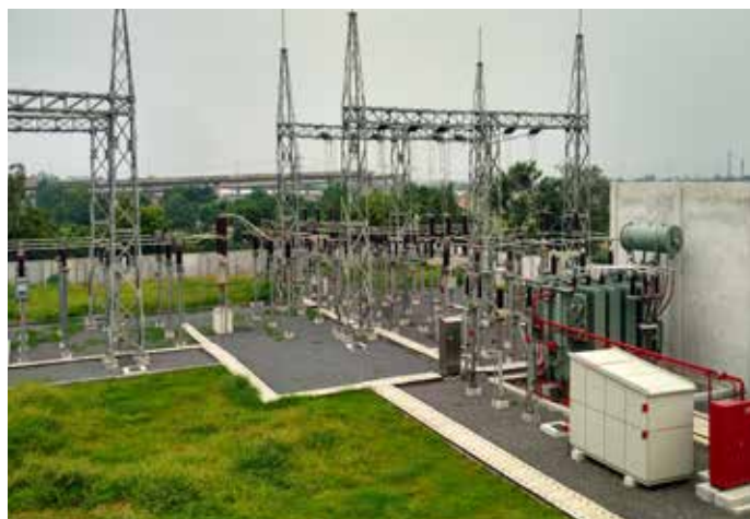
66 KV Yard at Mukundpur, Delhi
